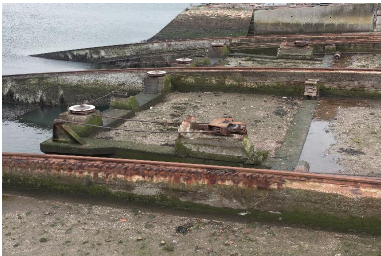
Rampes, rails, poulies, câbles
