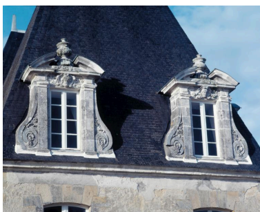
Château, pavillon sud-est. Elévation sud, lucarnes. Phot. Guy Artur, Phot. Norbert Lambart IVR53_19935602404XA
