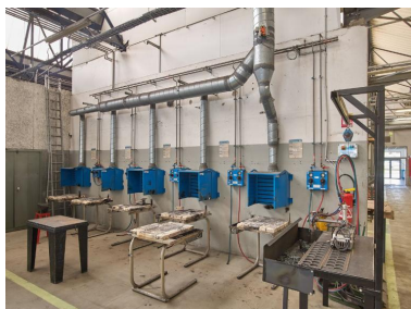
Atelier soudure. Phot. Bernard Bègne IVR53_20212900071NUCA
